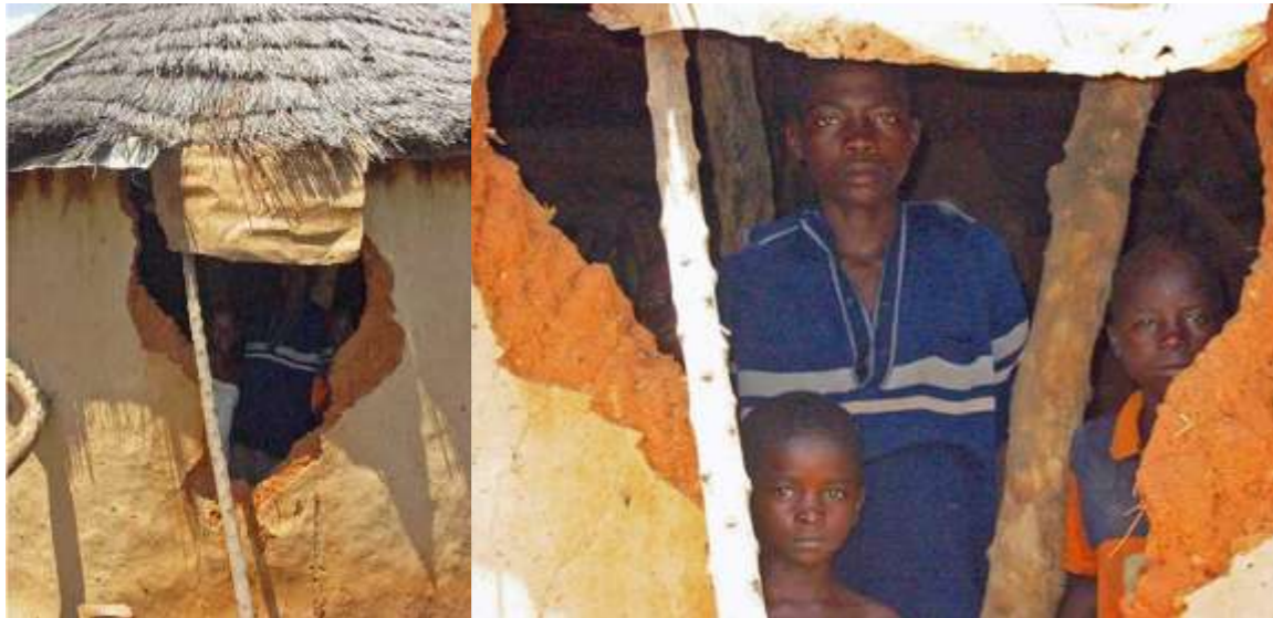
These children are wondering how much longer their round house will stand. Will the next rainstorm cause it to collapse? Notice their house is also being shored up with limbs. They also wonder if anyone will come to help. Kiteek, Northern Region
