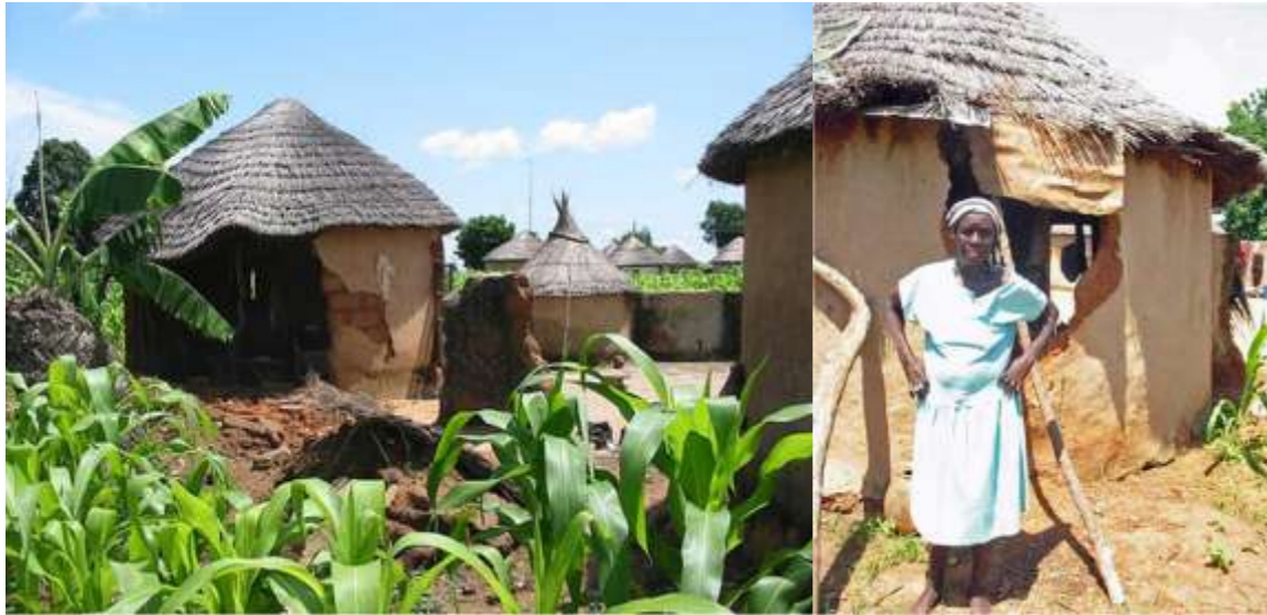
House in foreground completely collapsed. The 2nd house is heavily damaged and still occupied. Notice this elderly woman has the back of her house shored up with limbs. She is wondering if anyone will care enough to help. Will you? Kiteek, Northern Region
